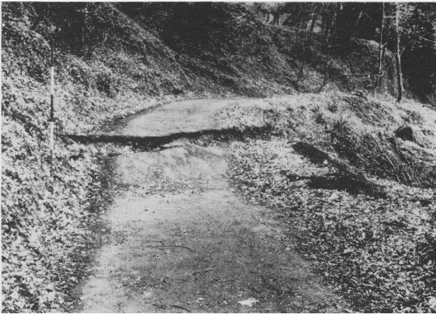
Figure 5: Disruption of the access road in February 1994 where crossed by the scarp at the base of block B (photograph taken on 7 March 1994).
